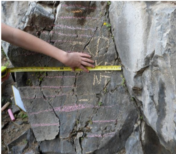
Figure 3: Column width being measured. Striae are marked with chalk.
